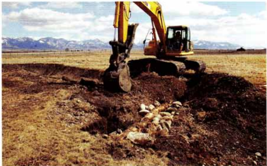
DIRT WORK. On a larger water reclamation project, reshaping a landscape may require as much as a full year of extensive planning as well as hands-on implementation by skilled personnel using heavy equipment.
